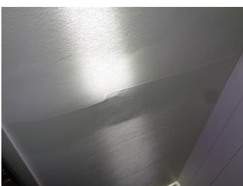
Wall cracked along sheet joint
