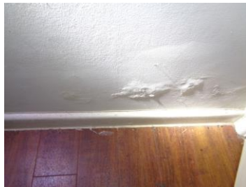
Wall behind door moisture affected
