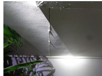
Wall cracked along sheet joint
