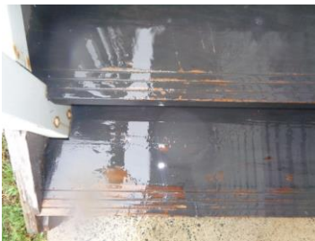
Stair tread paint finish worn
