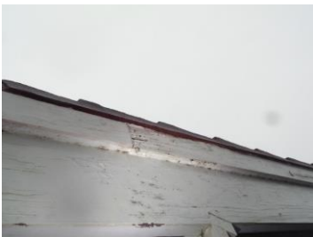
Barge board weathered
