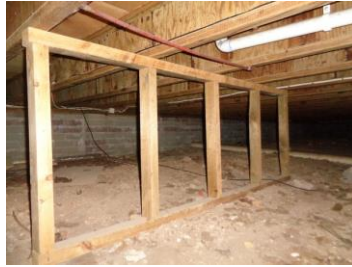
Timber support below kitchen can allow termite entry
