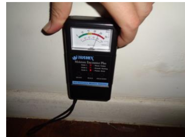
High moisture in wall
