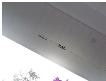
Veranda ceiling paint finish worn
