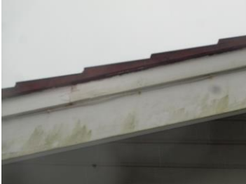
Barge board weathered
