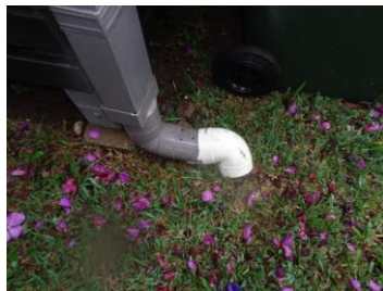
Downpipe not connected to stormwater
