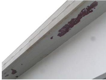
Gutter paint finish worn
