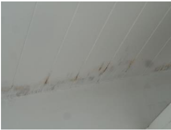
Eave lining water stained
