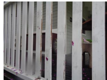
Veranda paint finish worn
