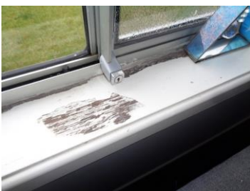
Window sill weathered
