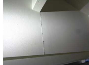
Wall cracked along sheet joint
