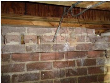
HWS overflow should be diverted
