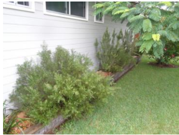
Foliage against the exterior can allow undetected termite entry
