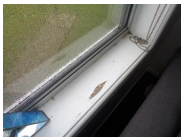
Window sill weathered
