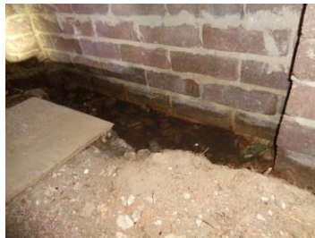
Water pools along the foundation wall
