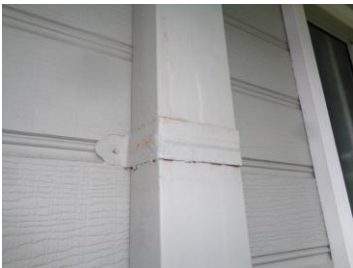
Downpipe bracket rusting
